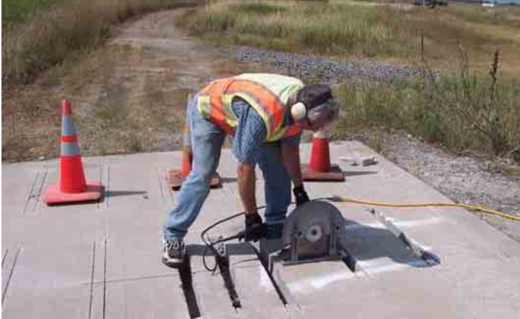
Figure 7. Saw cut being made on test slab to simulate a joint at the MnRoad facility.
