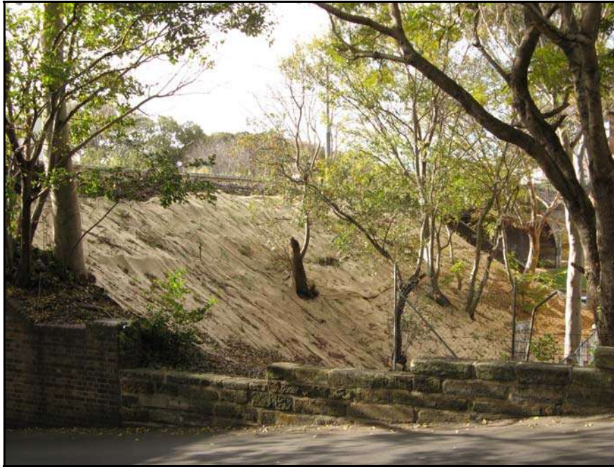
Figure 10. A recent revegetation project that has no habitat value for Superb Fairy-wrens. Light Rail Corridor between Bellevue Street and Wentworth Park Road. The Chinese Hackberry s trees have been left in situ and the slope otherwise cleared and replanted with Lomandras and Dianellas. This is currently probably good Currawong habitat. Enhancement plantings of dense shrubs and removal of Chinese Hackberry trees may be able to convert it to good Superb Fairy-wren habitat.
